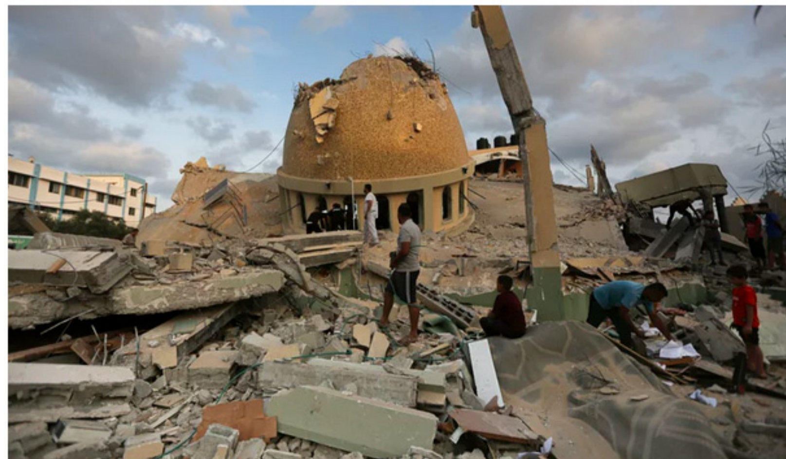
Israel says that artificial intelligence is allowing it to precisely target Hamas infrastructure. Independent researchers say roughly one in three buildings in Gaza have been damaged or destroyed.
