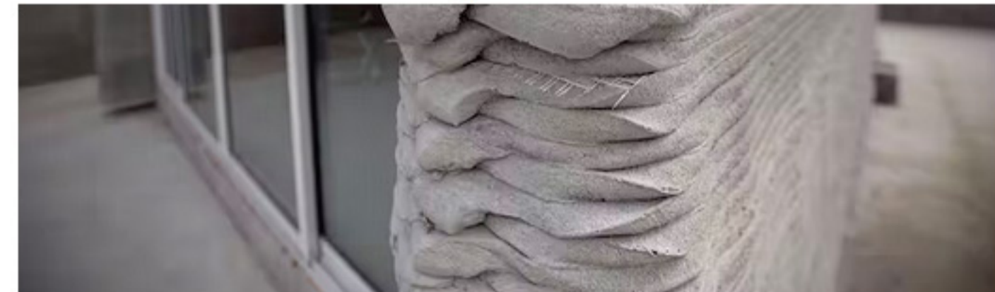
A 3D-printed house in Shanghai that was built in less than 24 hours out of construction waste. Visual China Group/Getty Images
