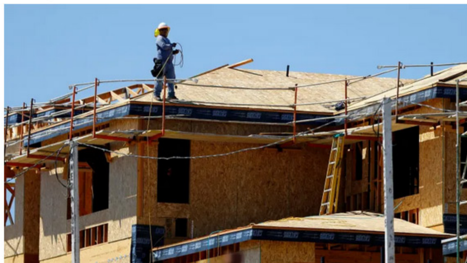
A worker walks on the roof of a new home under construction in Carlsbad, California.
