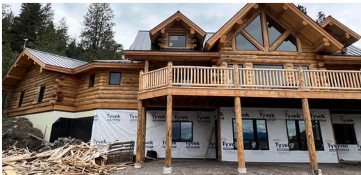
Steve Holett worked 12 to 15 hours a day to build their home for retirement.
