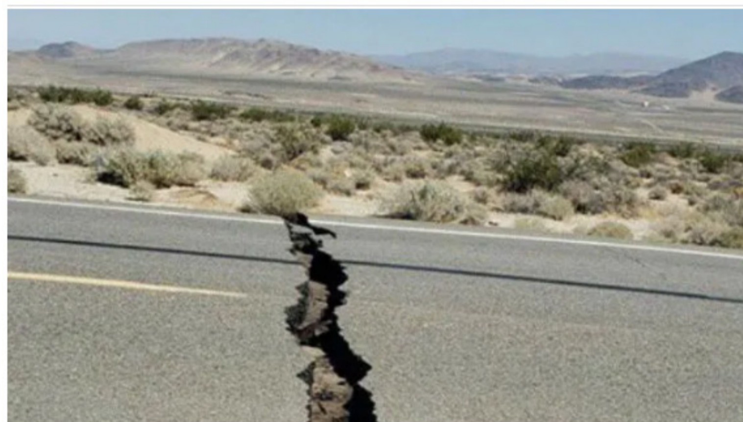
Damage from a 6.4-magnitude quake near Trona on July 4, 2019. Courtesy Caltrans
