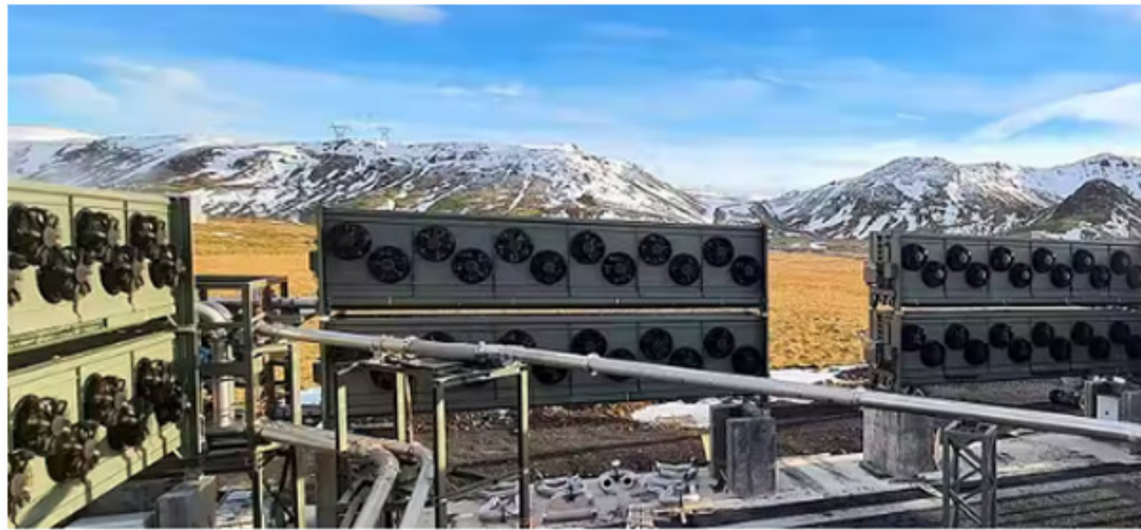
This direct air capture plant in Iceland was designed to capture 4,000 metric tons of carbon dioxide per year. Climeworks 2021 via AP Photos
