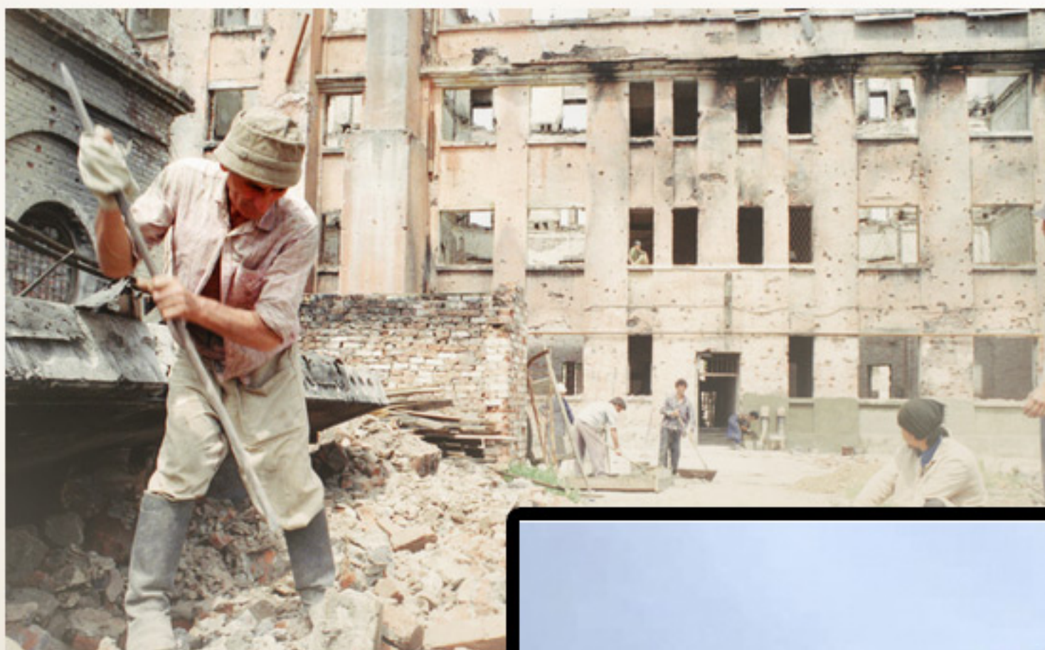
Residents of Grozny dig through rubble of destroyed buildings to salvage whole bricks to repair their destroyed houses following the siege and takeover by Russian forces this year in Grozny, May 26, 1995.
