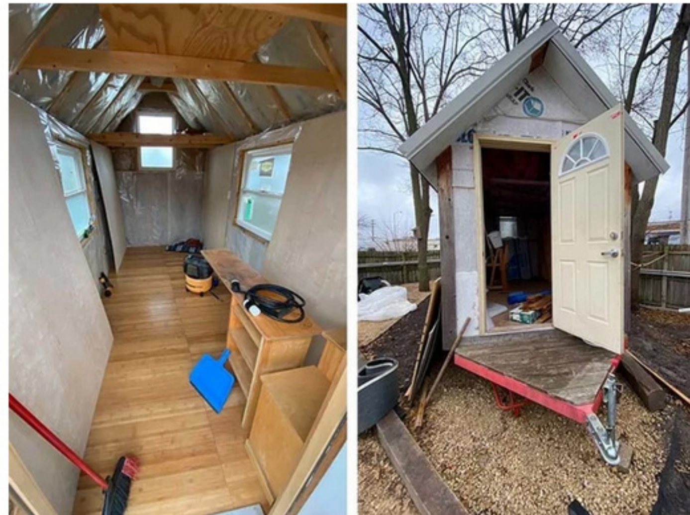
Interior and exterior views of a home under construction in a tiny home village operated by Occupy Madison in Madison, Wisconsin, December 2021.
